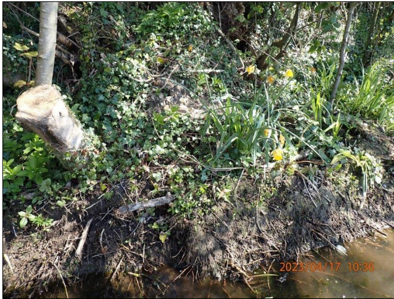
Photograph 7. (Exhibit AM01G-P4170009) Reprofiling of left bank of bypass channel and disposal of gravels (behind daffodils) on bank.
