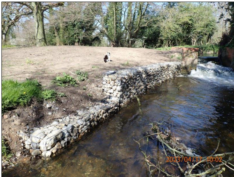
Photograph 6. (Exhibit AM01F-P4170001) Gabion baskets installed along right bank of mill bypass channel.
