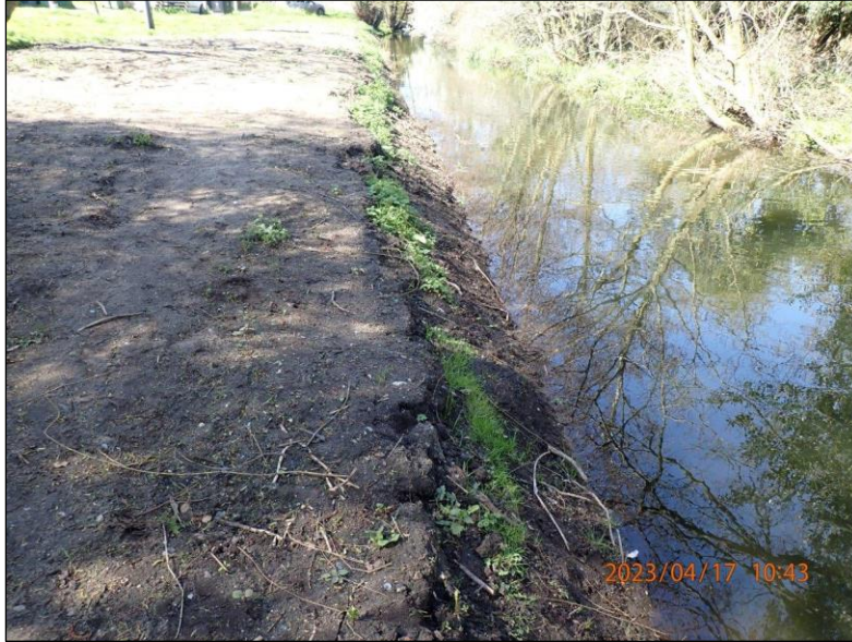
Photograph 1. (Exhibit AM01A – P4170012) General view of affected reach showing spread spoil and reprofiled river bank.
