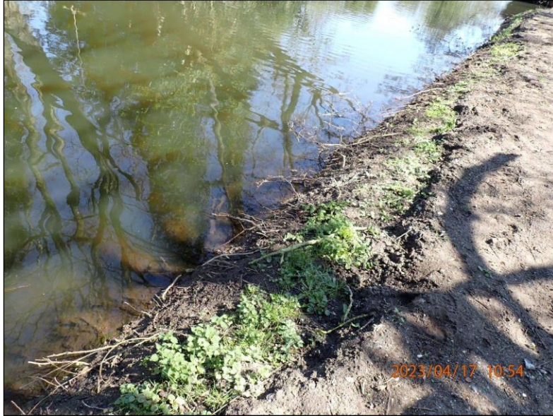
Photograph 3. (Exhibit AM01C-P4170016) Reprofiled bank edge showing cut through reed rhizomes/plant roots.
